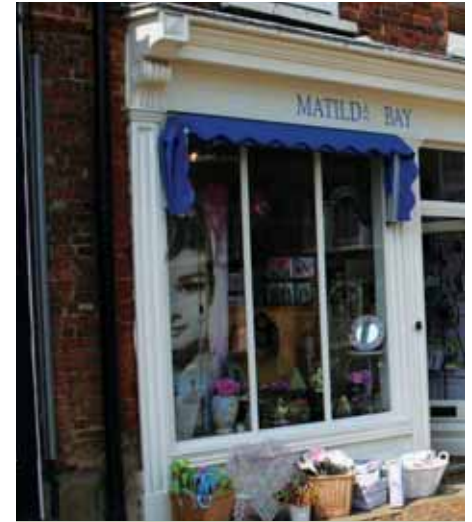
Fig 11 Pilaster are an important part of the shopfront and often 'contain' the fascia at both ends (Woburn)
