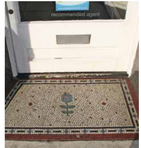
Fig 12 Decorated thresholds add interest to the shopfront and should be retained/restored or reinstated wherever possible (Biggleswade)
